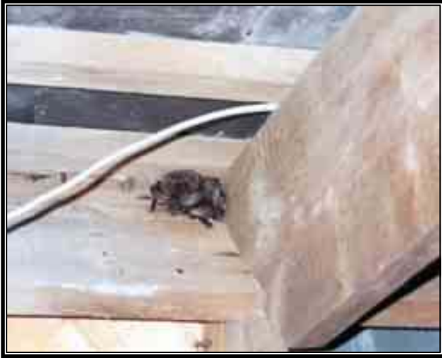
Figure 6 Grey long eared bats roosting at the junction of rafters and roof batons in July 2001.
